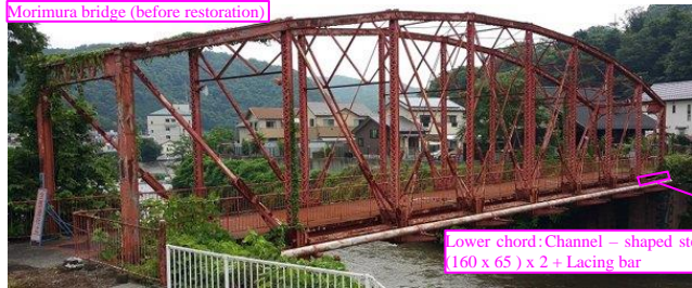
Morimura bridge (before restoration)
