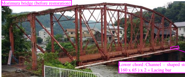
Morimura bridge (before restoration)
