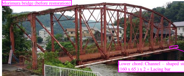
Morimura bridge (before restoration)
